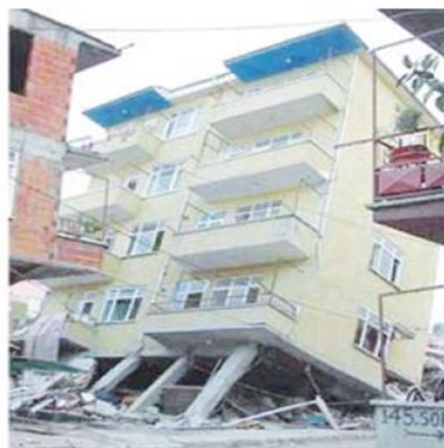
Figure.1 Soft storey failure in Tukery
